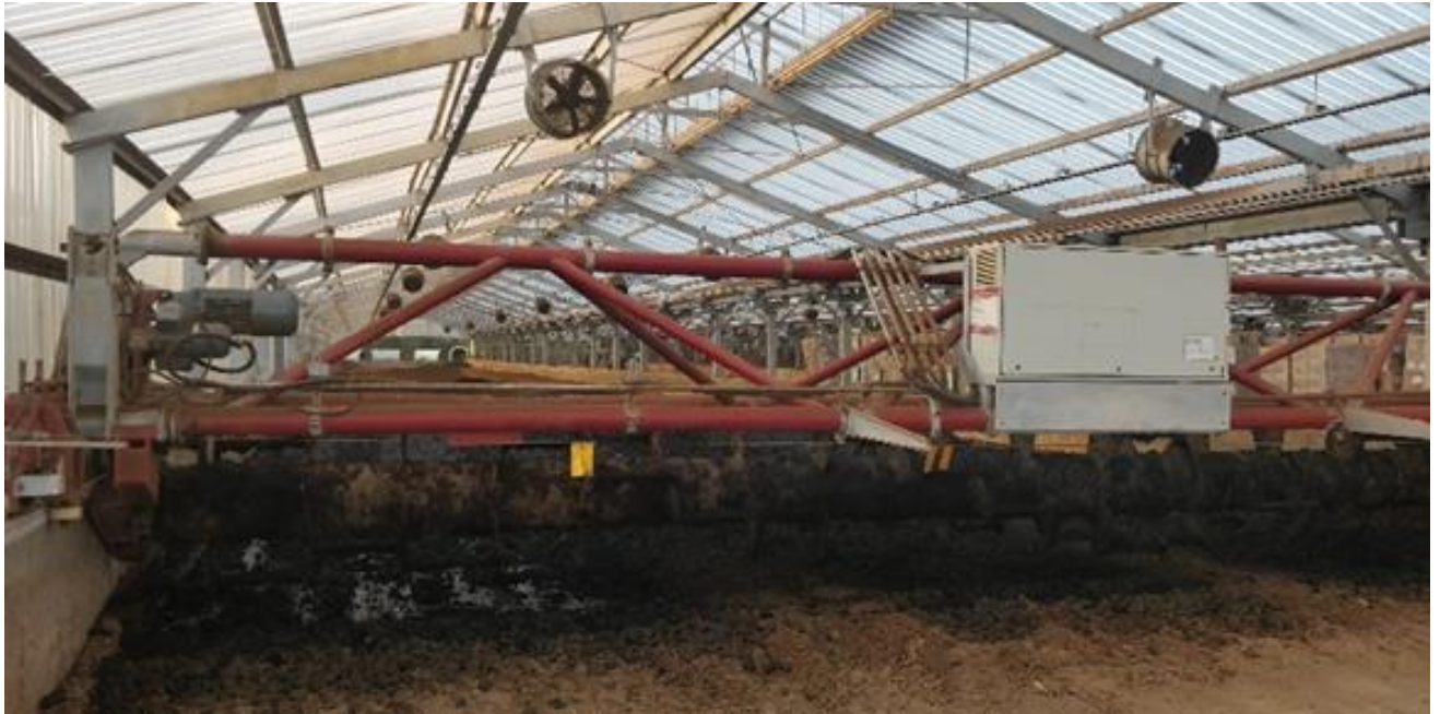
Figure 4-1: Solar Thermal Sludge Drying unit in Surat, India
